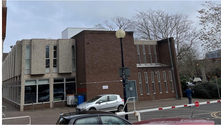
Figure 7: existing library rooftop plantroom that might be adapted to house heat pump plant
