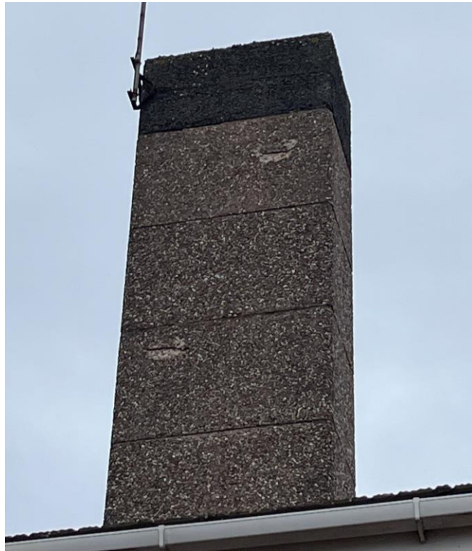
Figure 1: existing boiler flue showing concrete damage
