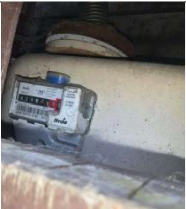
OUTSIDE GAS METRE
